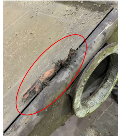
Figure 4b. Impurities in blowing slots
