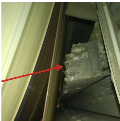
Figure 5a. Damaged physical sealings
